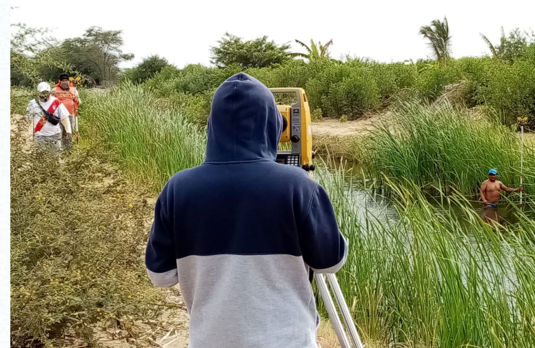
Hired Sub-Consultant (Luis Solis + Team) Conducting Topographic Land Survey in Las Mercedes KM11 to be used in the Clean Water Solution Design. (2021-09-20)
